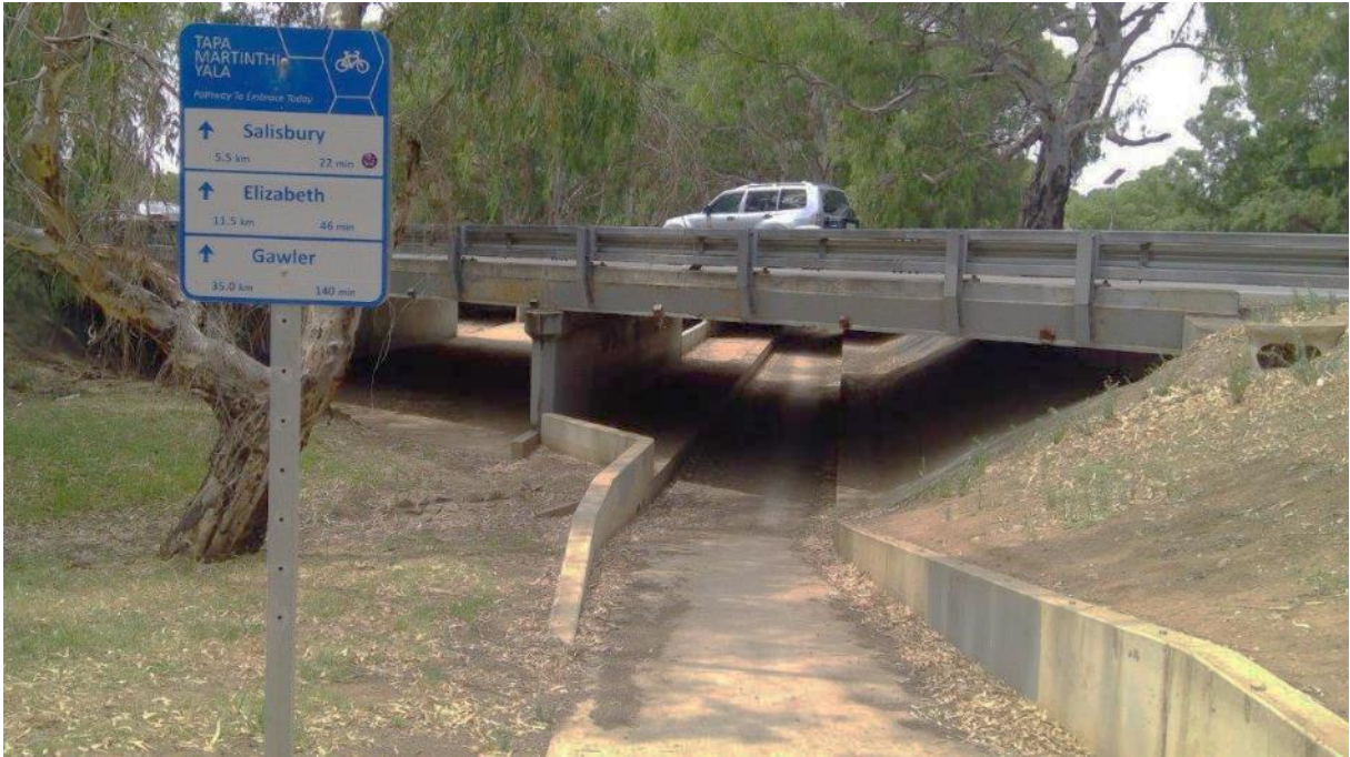
Figure 67: The Underpass of Port Wakefield Road regularly floods and fills with debris
